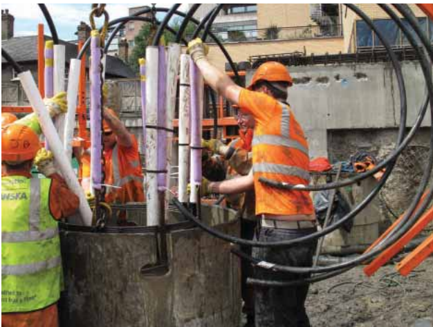
Geothermal loops being installed on the cage going in to the pile at the London Bankside project.
